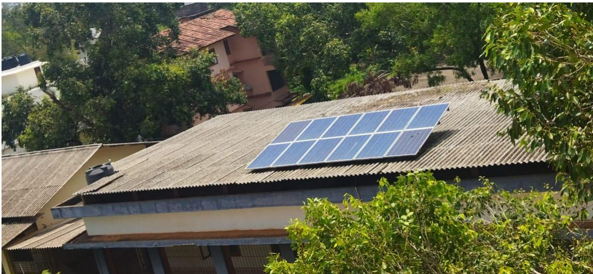
FIGURE 14: SOLAR INSTALLATION - MATHS BLOCK
